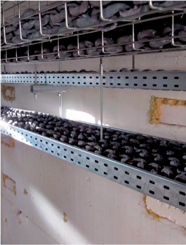
Cable tray with high mechanical load before...
